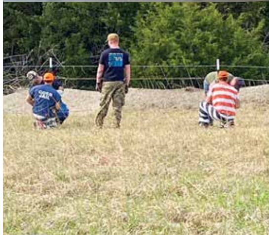
Inmates who volunteered for the job helped with construction on every phase of the project.
